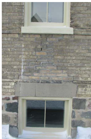
East elevation, showing detail of cracked concrete lintel and cracked and open mortar joints (ERA, 2019).
