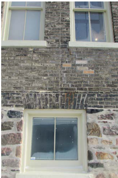
West elevation stone foundation and basement window, showing cracked mortar joints above window (ERA, 2019).
