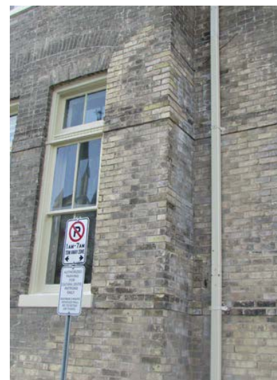
East elevation, showing area of efflorescence (ERA, 2019).
