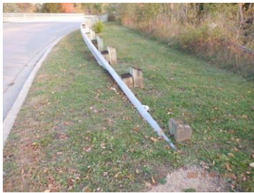
Substandard Buried End Treatment
