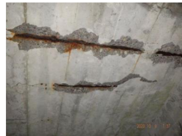
Spall and Delamination with Exposed Reinforcing Steel
